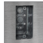
TA-62F Empty Junction Box
